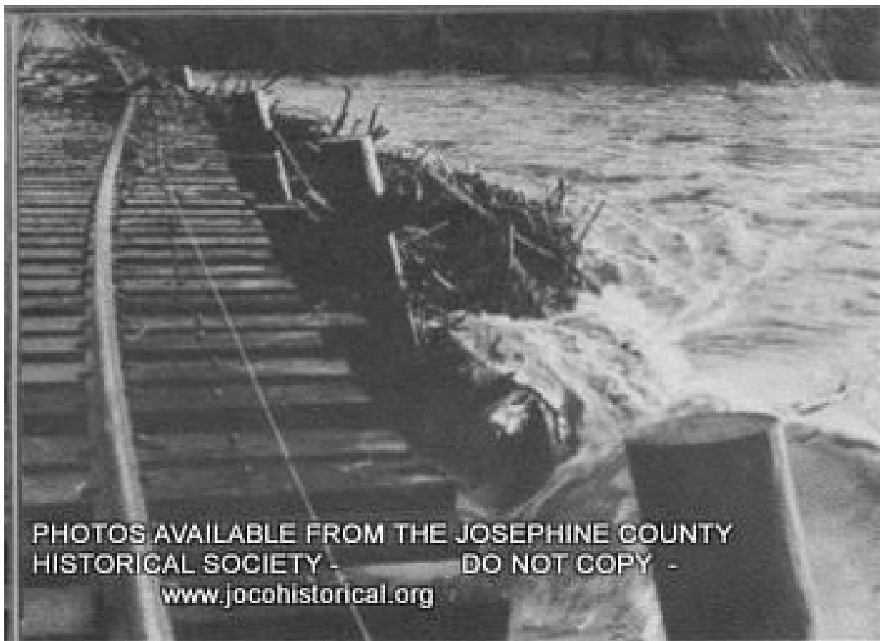
Applegate RR Bridge debris
